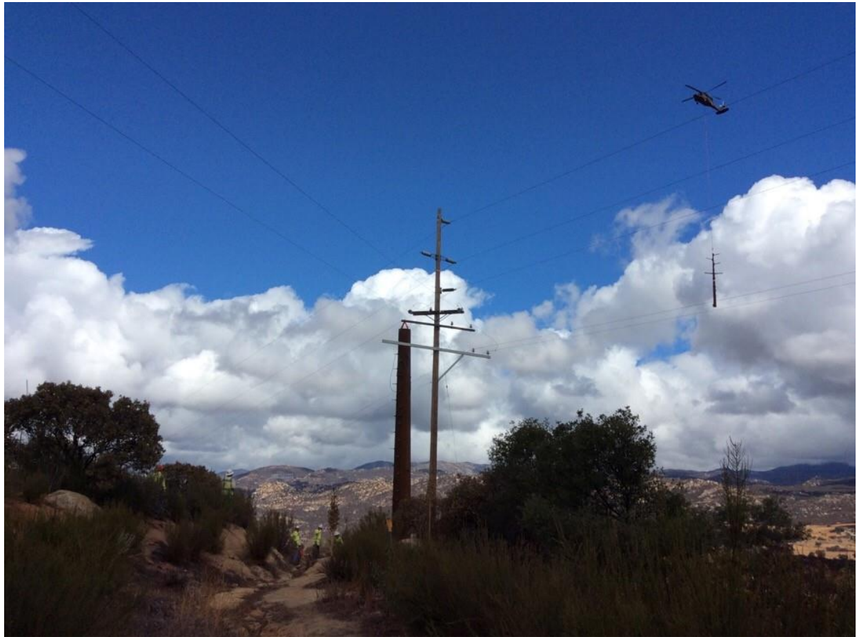
Photo 2: A crew observed installing a new steel pole top at Pole Z571421 (TL 6957).
