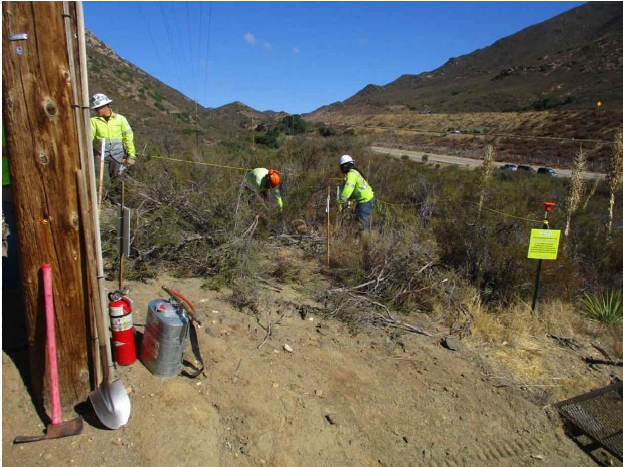
Photo 4: During vegetation clearing at Pole Z40510 (TL 629C), the construction crew staged a set of fire tools within 50 feet of work activities in accordance with the CFPPP, MM FF-1, and MM HAZ-04. The work space was surrounded by a ESA (rope and signage) and archeological and Native American monitors were present on-site during work activities in accordance with the Historic Properties Management Plan (HPMP), MM CUL-1, APM CUL-03, and APM CUL-04, and APM CUL-05.
