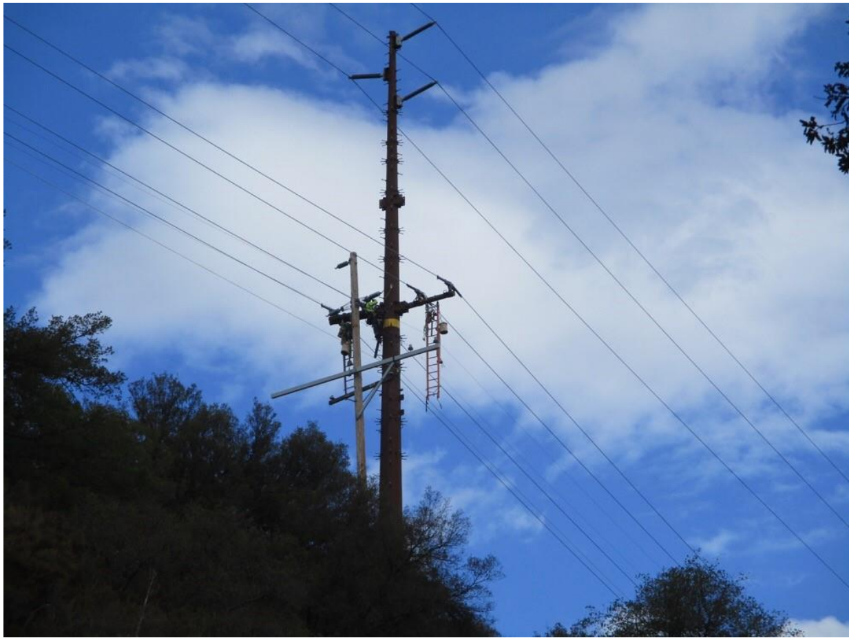
Photo 1: A CPUC ECM observed a wire stringing construction crew dead-ending new 12 kV conductor wire at Pole Z118111 along TL 682.
