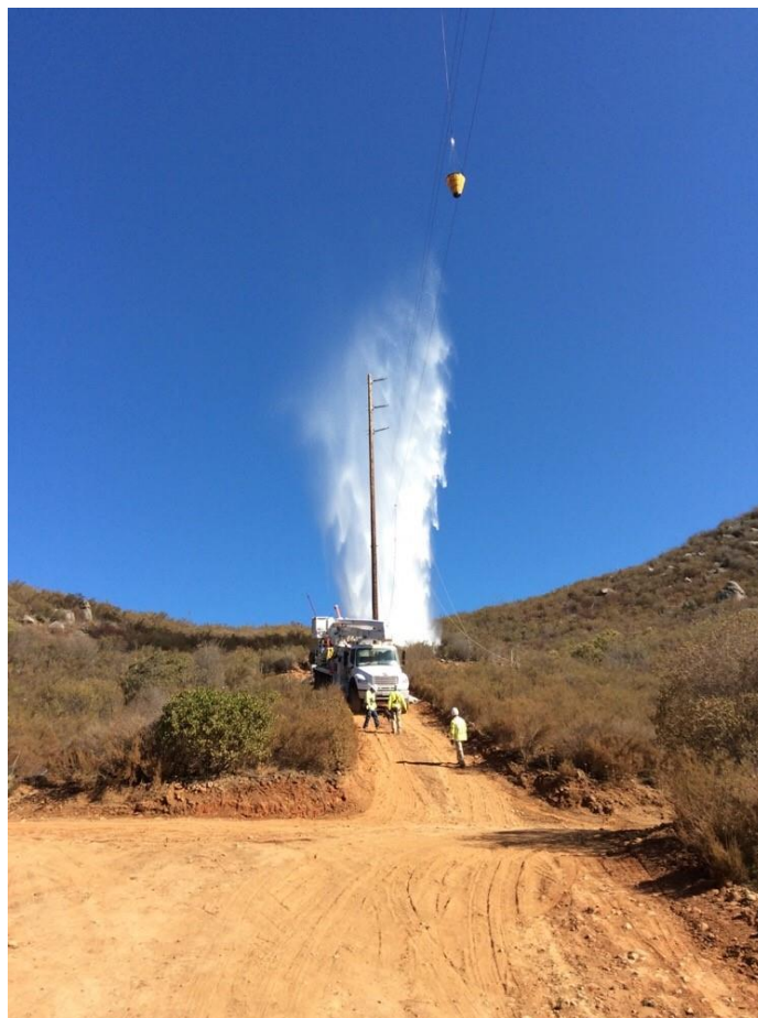
Photo 5: In order to minimize dust emissions from helicopter rotor wash during pole setting at Pole Z571449 (TL 6957), water was dropped on the site prior to pole delivery in accordance with APM AIR-05.
